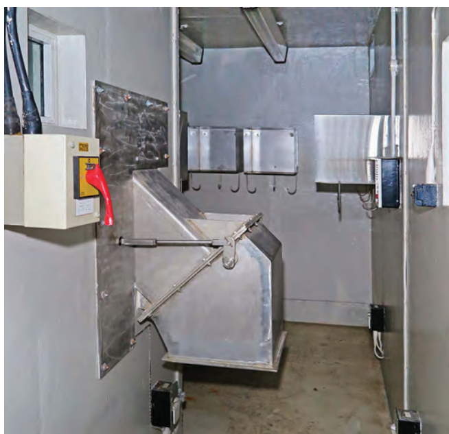
Chute for disposing of contaminated clothing in the decontamination area. Photo Clive Penfold
